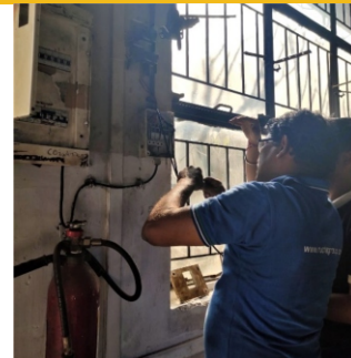
Pic: Manual process of activating and deactivating fans
